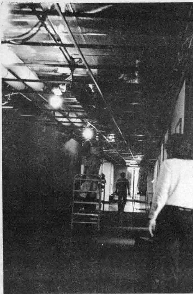
THE SKY IS FALLING: Technicians work on the framework of the ceiling in SSB in an effort to contain a water leak [photo by Dale Nelson].
